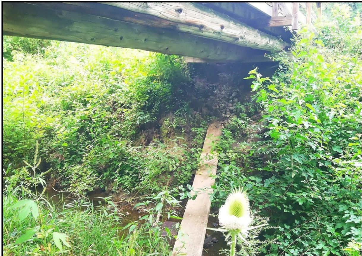
Photo: Erosion at Fuller Park
