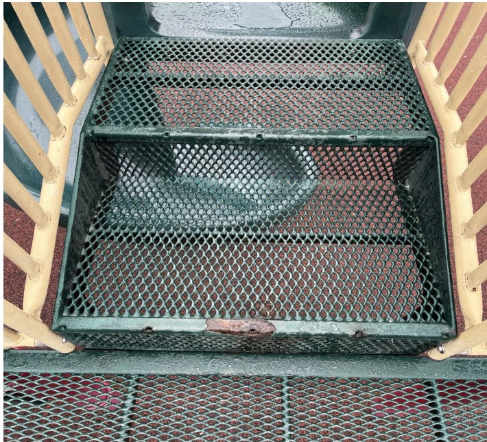
Platform surface to be replaced
