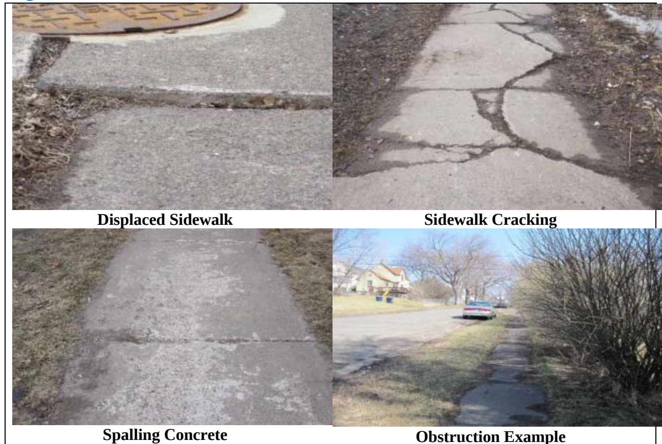
Figure 1: Sidewalk Surface Deficiencies 5
