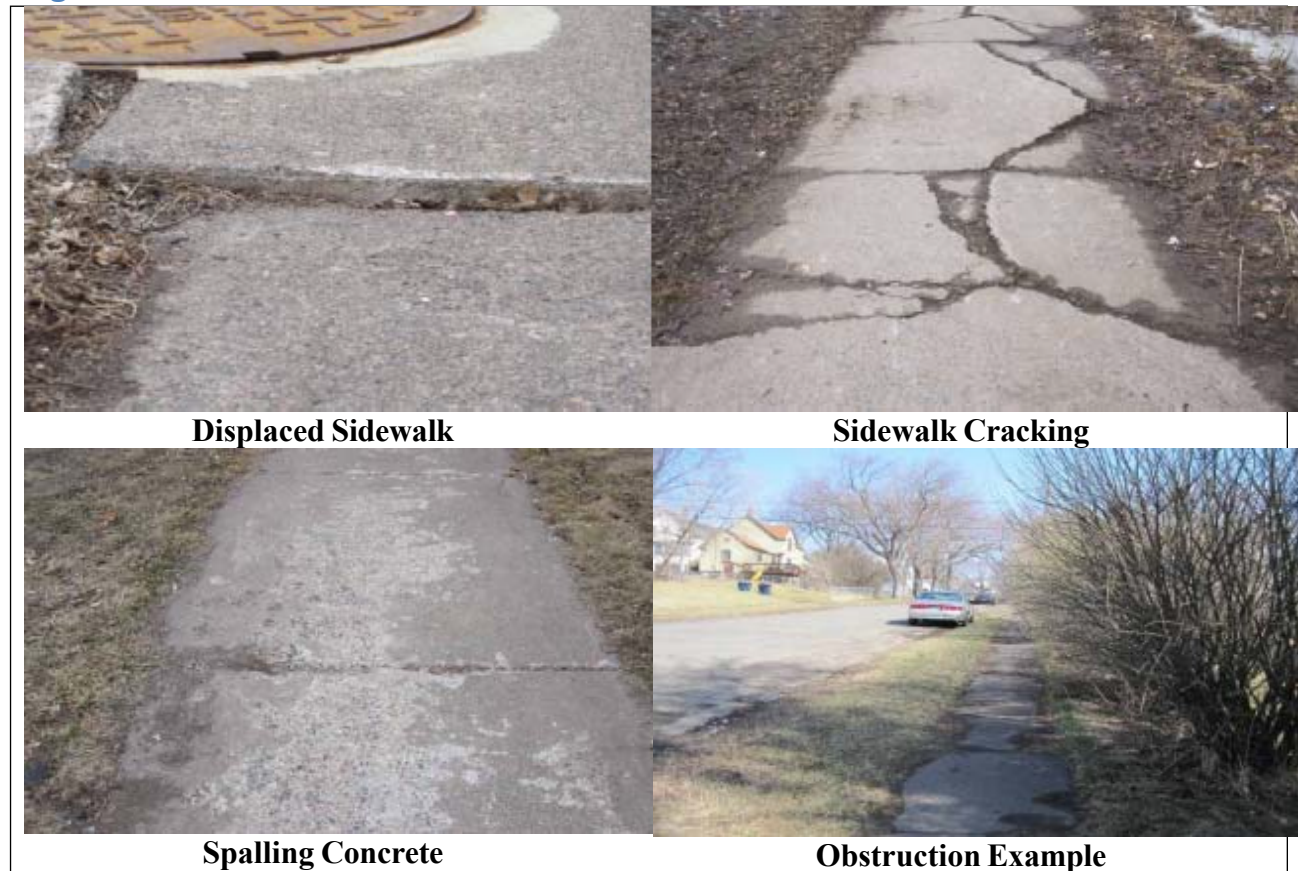
Figure 1: Sidewalk Surface Deficiencies
