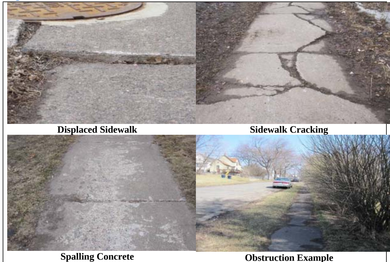
Figure 1: Sidewalk Surface Deficiencies 5
