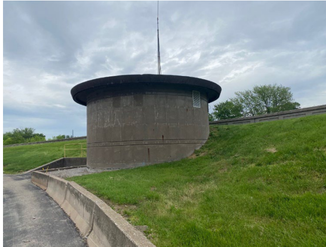
Figure 3-6: Exterior of Mad Creek Lift Station
