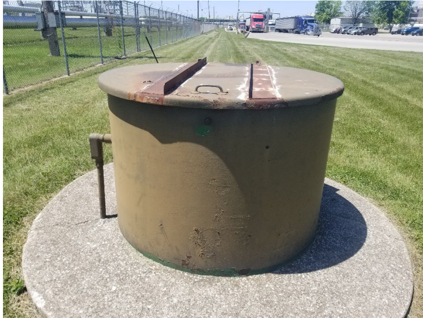
Figure 3-27: Exterior of Maple Grove Lift Station
