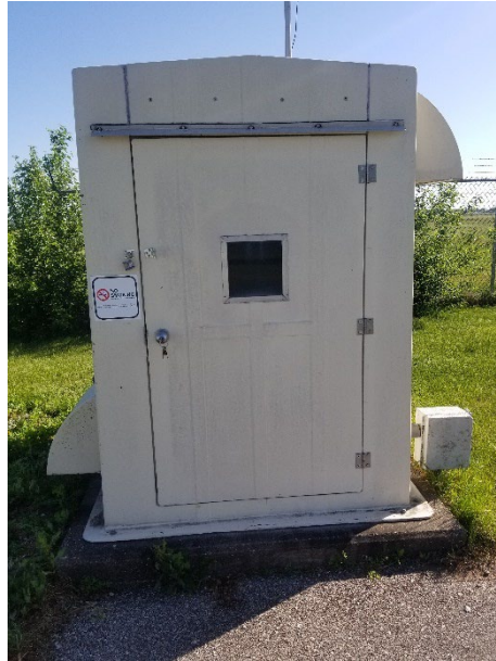
Figure 3-24: Exterior of Airport Lift Station
