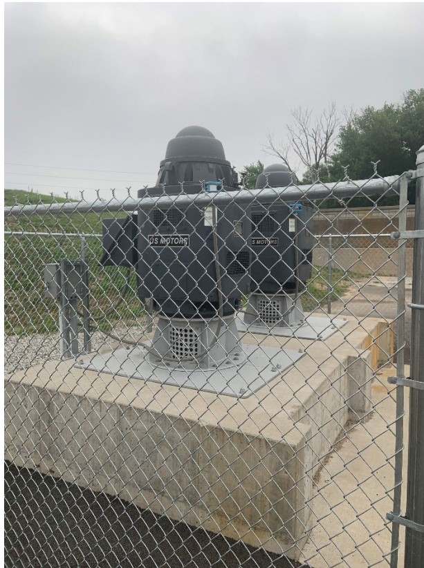
Figure 3-25: Exterior of HNI Stormwater Lift Station
