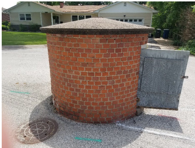
Figure 3-26: Exterior of Magnolia Lift Station
