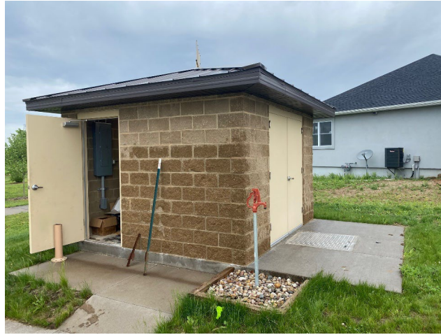
Figure 3-9: Exterior of Arbor Commons Lift Station
