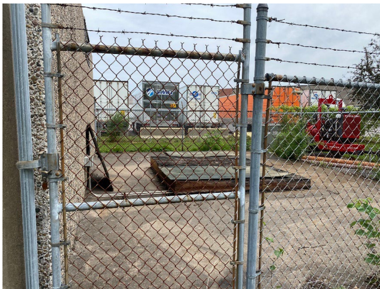
Figure 3-23: Isett Wet Well Cover
