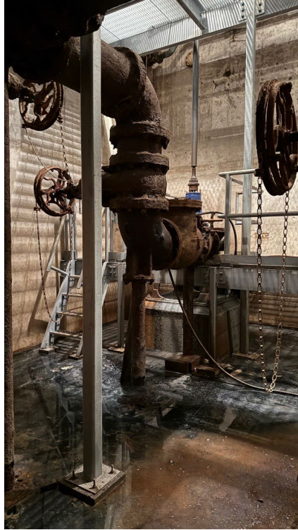
Figure 2-9: Process Pump and Piping
