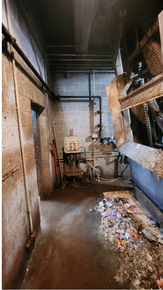
Figure 2-7: Bar Screen Room
