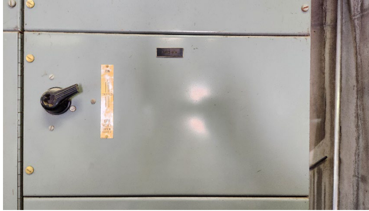
Figure 2-2: Broken Breaker Handle
