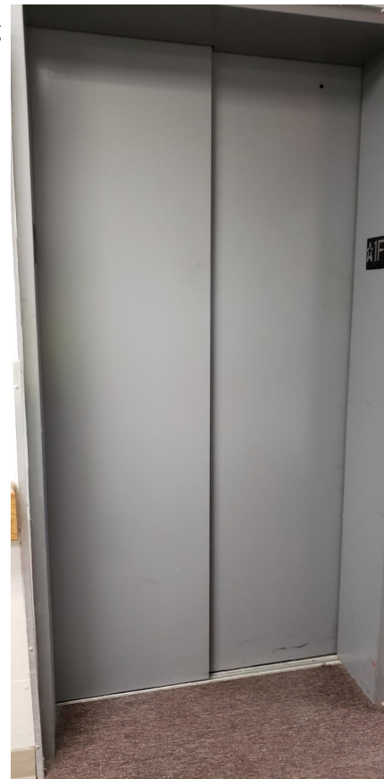
Photo: Current Clark House Elevator
