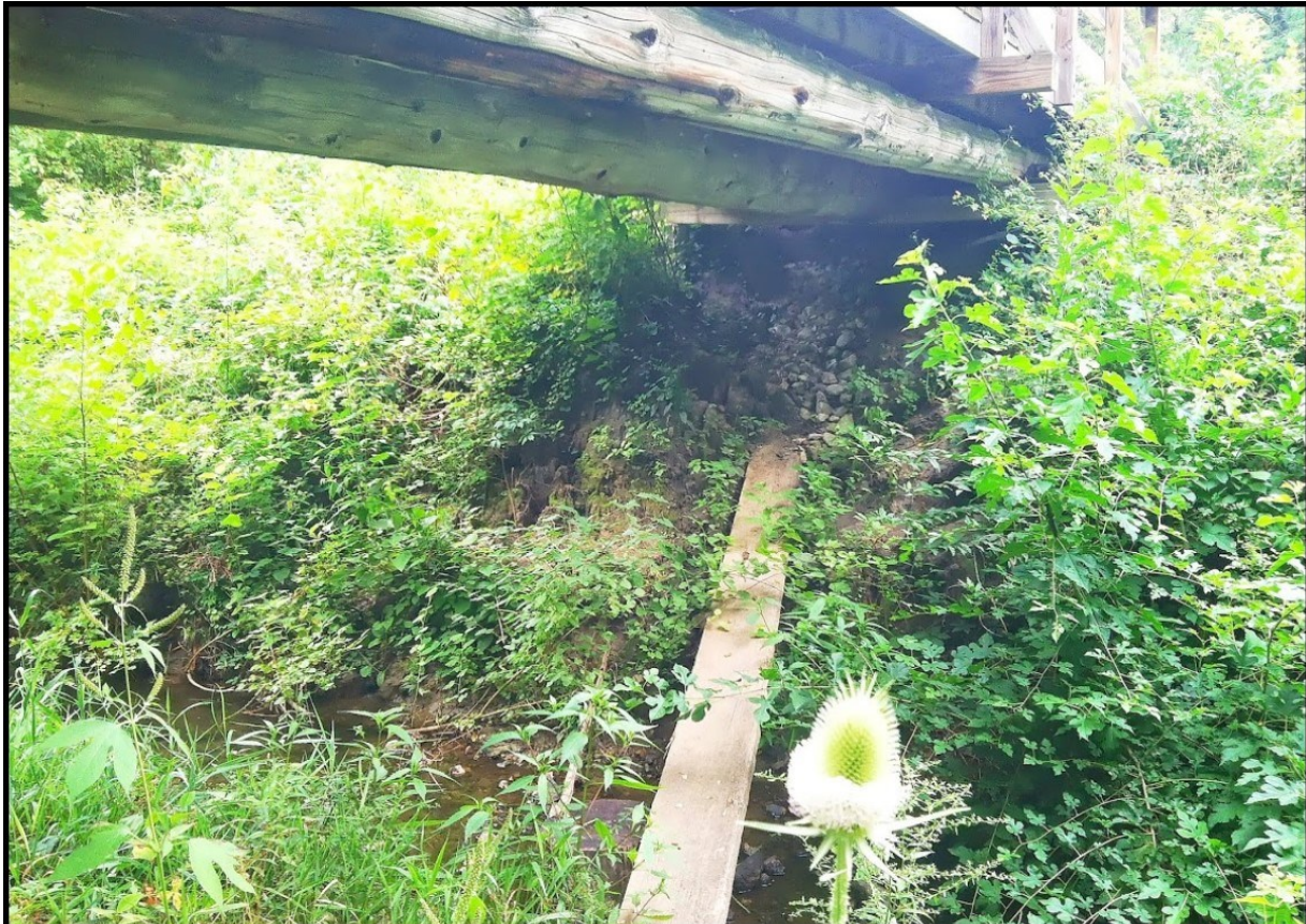
Photo: Erosion at Fuller Park
